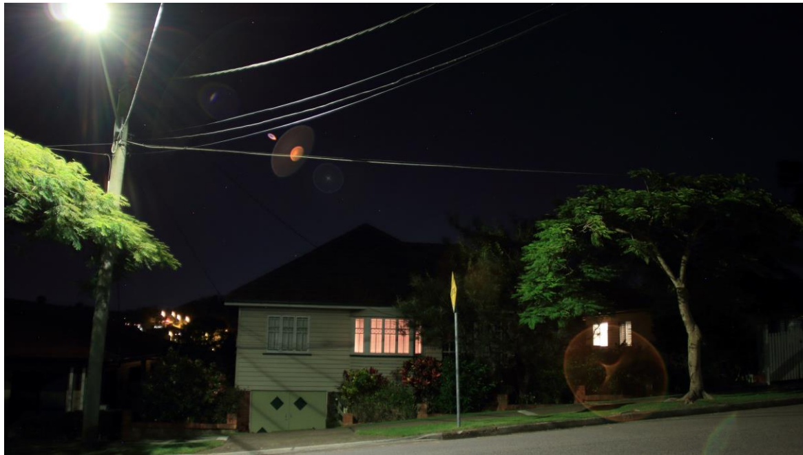
This luminaire delivers a very wide field of illumination and substantial rear light trespass.
