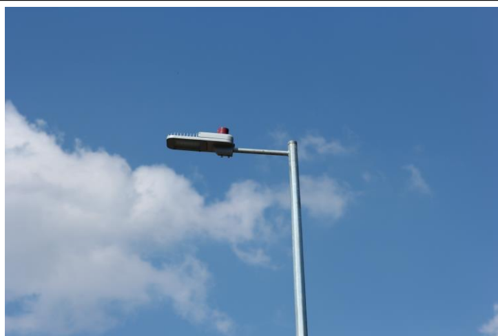
An example of up-tilted LED luminaire installation in the western end of Galleon Street, Jamboree Heights.
