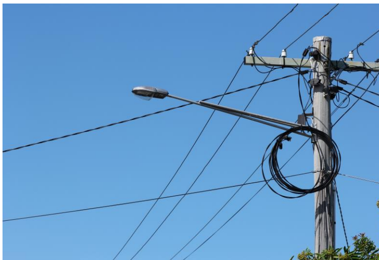
Almost all the trial luminaires in this street are installed with an up-tilt, some by as much as 10°.
