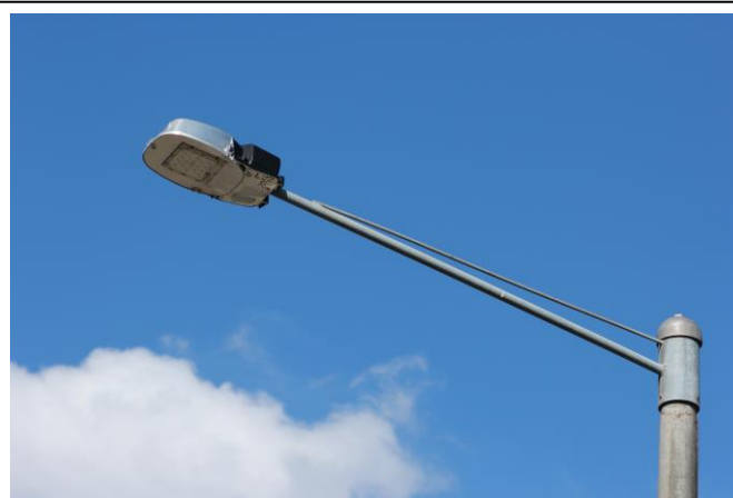
All of these trial luminaires in the eastern end of Malbon Street are installed with an up-tilt angle of at least 5° and some are up-tilted substantially more.
