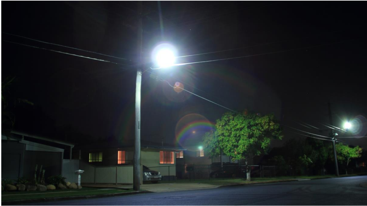
Substantial rear light trespass from this luminaire.
