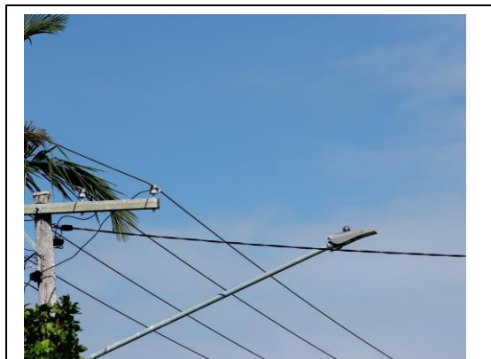
Luminaire with up-tilt estimated at greater than 10°.
