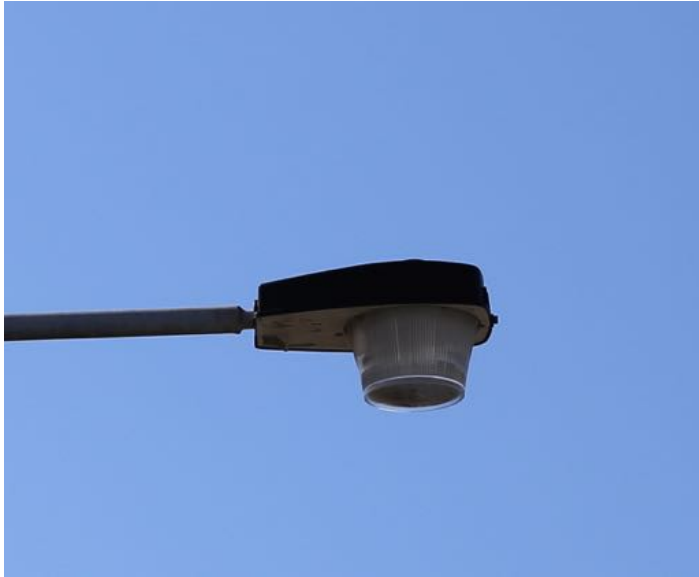
Figure 13. Unshielded Mercury vapour luminaire (Author's Personal Photo).
